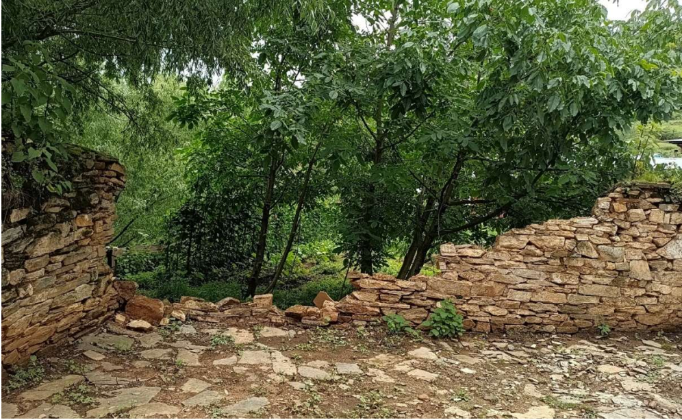
The collapsed wall
